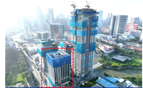
Redevelopment of former Somerset Liang Court Singapore Expected completion in 2026 and opening in 2027
